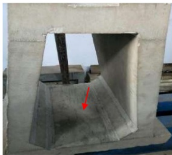
Fig.13: Side wall – bottom crack foundation
